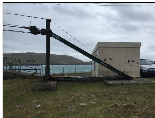
Plate 14.12: Island-side cableway machinery and line station
